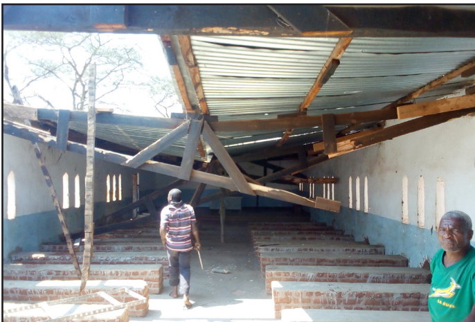
St. Matthew's with the new stone and concrete bench seating—yet major problems with the roof.
